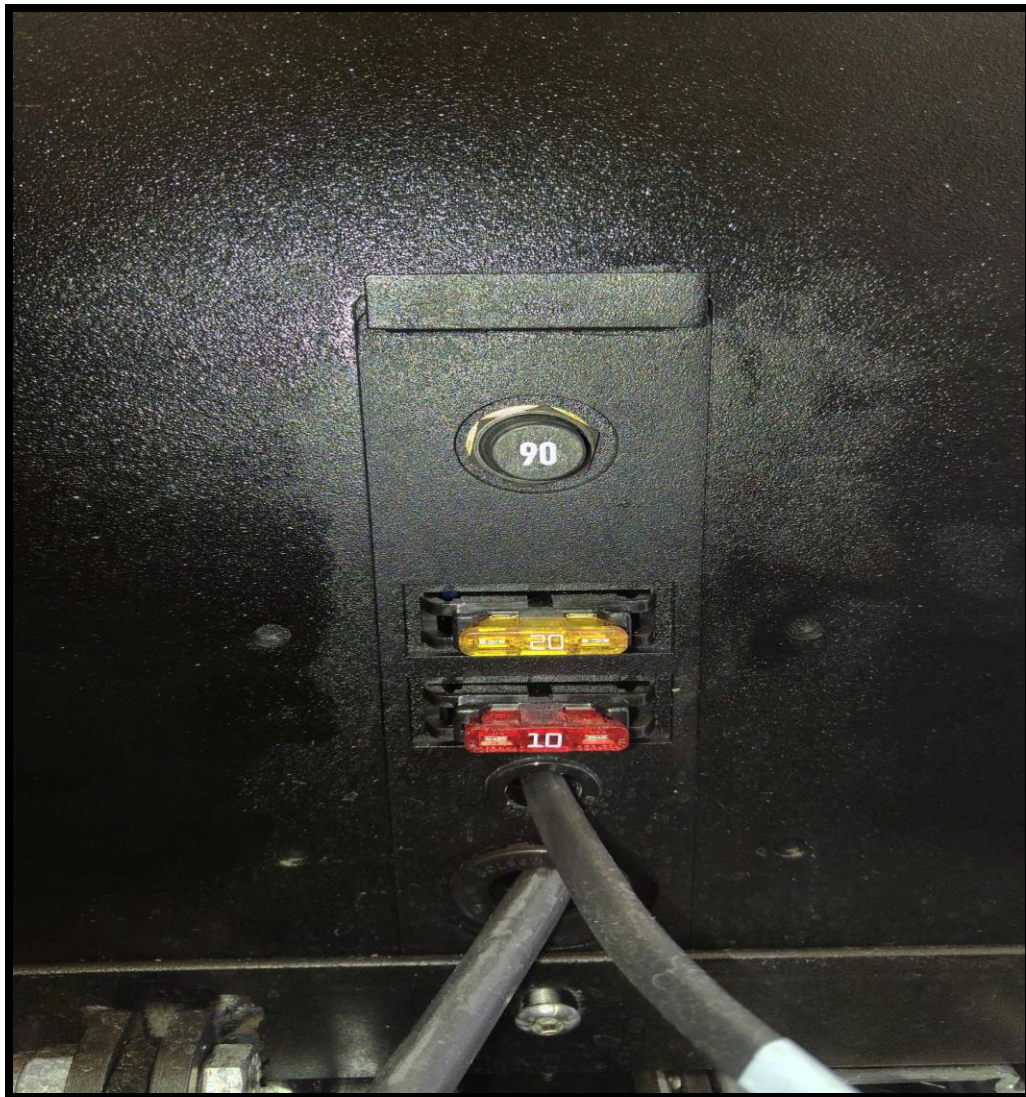
Top- 90 Amp Circuit Breaker (Pull for a "Hard Re-Set") Yellow Blade- 20 Amp Blade Fuse Red Blade- 10 Amp Blade Fuse
