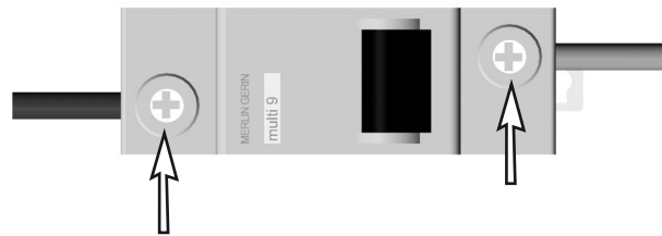
Main fuse cable connection.
