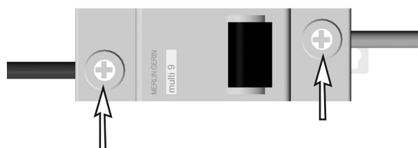
Main fuse cable connection.
